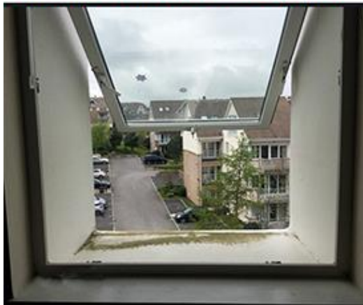
Without Window Restrictor-DANGER
